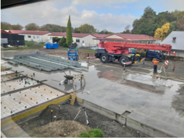
May 2021 - The concrete foundations have been poured and walls are beginning to take shape. The old NMIT reception has been moved off Ballinger Drive.
